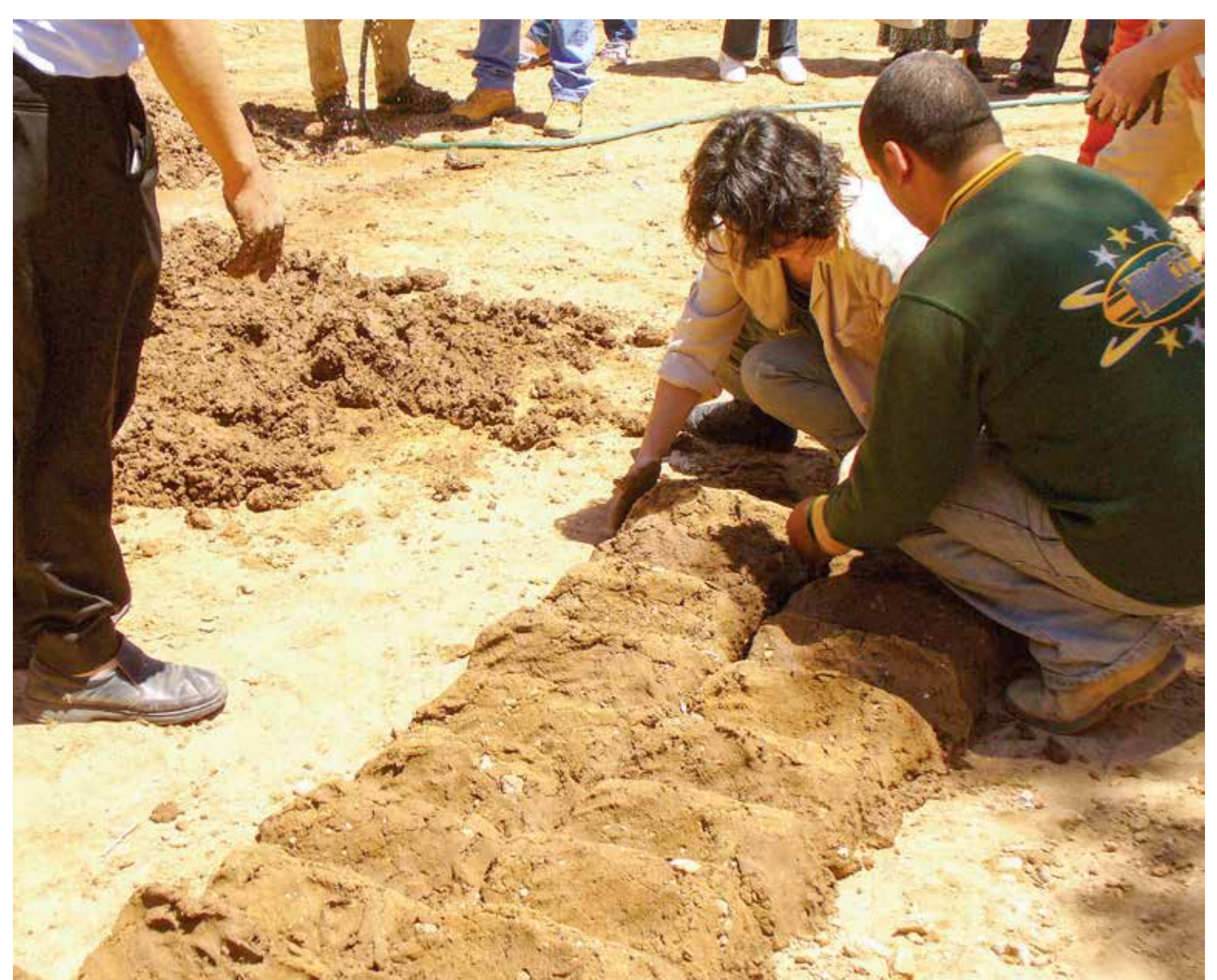
Fig.6 International experts learning how to prepare adobe building culture in Figuig, Morocco
